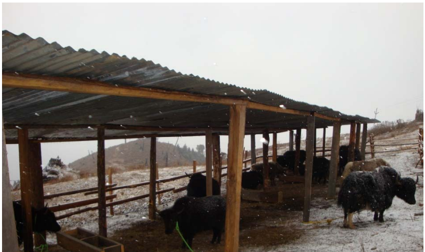
Yak sedentarization programme was successfully implemented at Mandala (10000 ft above msl) in 2011
